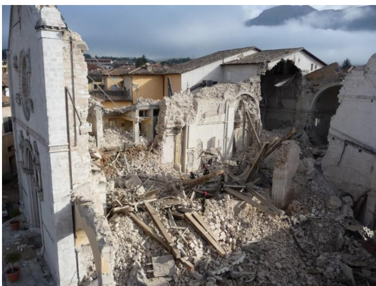
Internal view of the Basilica of San Benedetto in Norcia after the seism of 30 October 2016 © MiC
