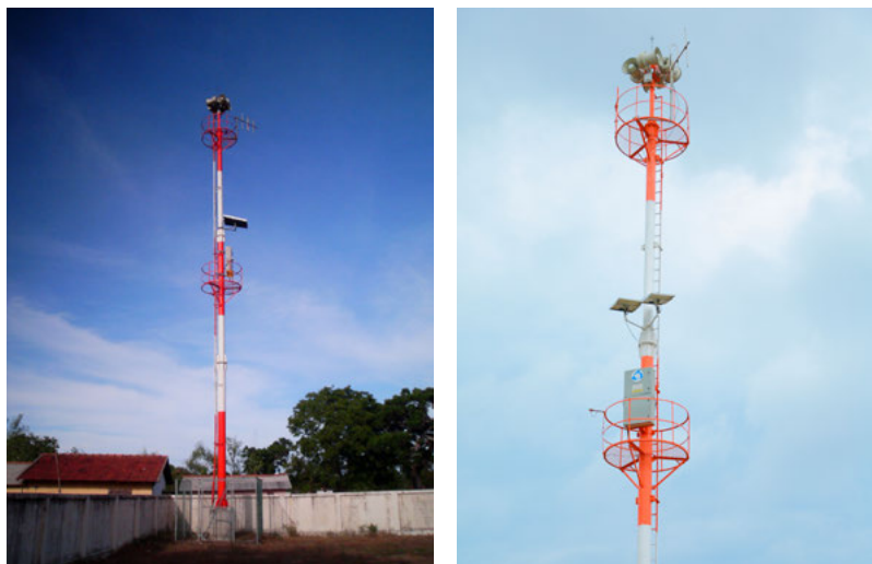
Figure 7.4 Tsunami warning towers, which consists of satellite communication, sirens, and solar power systems, erected along the Sri Lankan coastal belt
