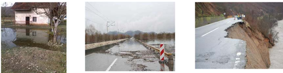
Figure 6.8: Flooded residential building in Bijelo Polje municipality (2010), the damaged road in Bar and Berane municipality (2010) (MPPFR Bijelo Polje, 2013; MPFPR Bar, 2019; MPPFR Berane, 2014).
