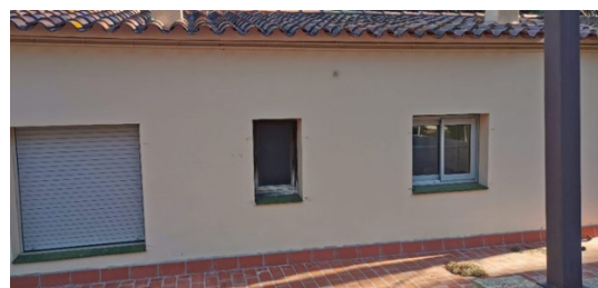
Figure 4: Unprotected glazing of the flat
