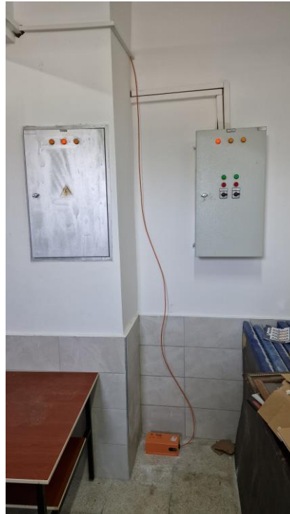
Figure 45. Cevatpaşa Ortaokulu Basement Floor Accelerometer Location (Instrumentation).
