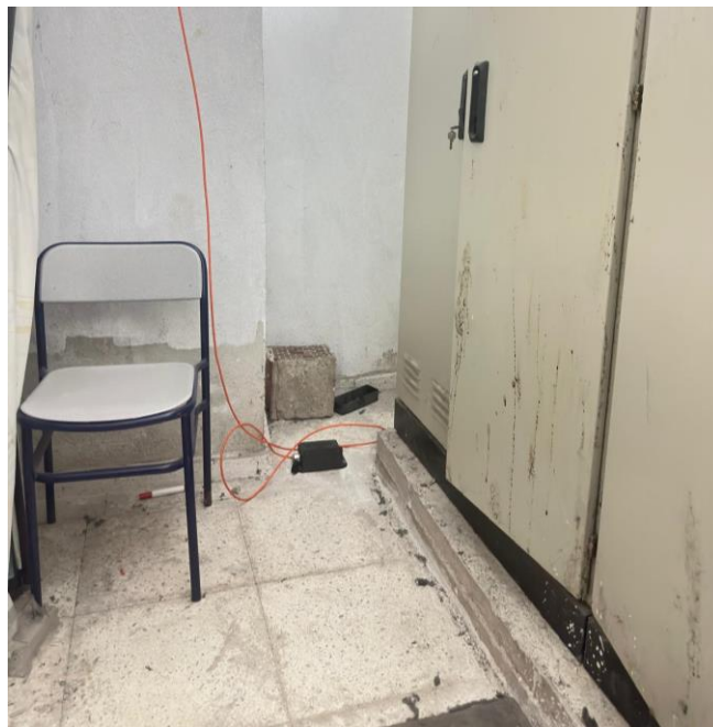
Figure 36. Prof. Dr. Aziz Sancar Ortaokulu Basement Floor Accelerometer Location (Instrumentation).
