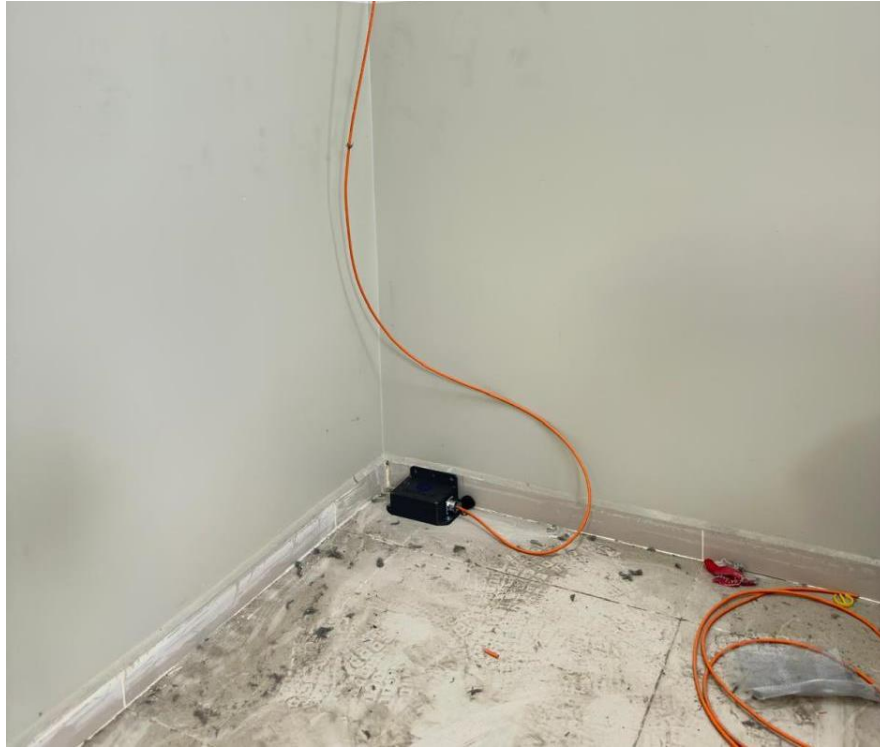
Figure 31. Bornova Anadolu Lisesi G-Blok 2 nd Floor Accelerometer Location (Instrumentation).
