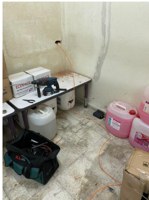
Figure 28. Ali Osman Konakçı Mesleki ve Teknik Anadolu Lisesi Basement Floor Accelerometer Location (Instrumentation).
