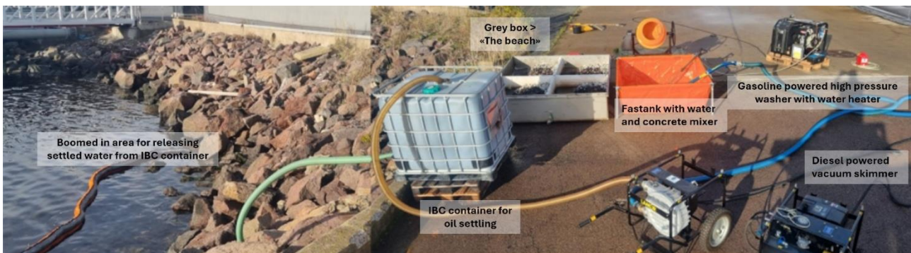
Figure 81: Example of a “sealed off” in-situ washing station: high pressure washer with heater, concrete mixer for tumbling/washing, vacuum pump skimmer for skimming the washing pool and an IBC container for collecting washed out oil from the pool and for settling of water /oil.
