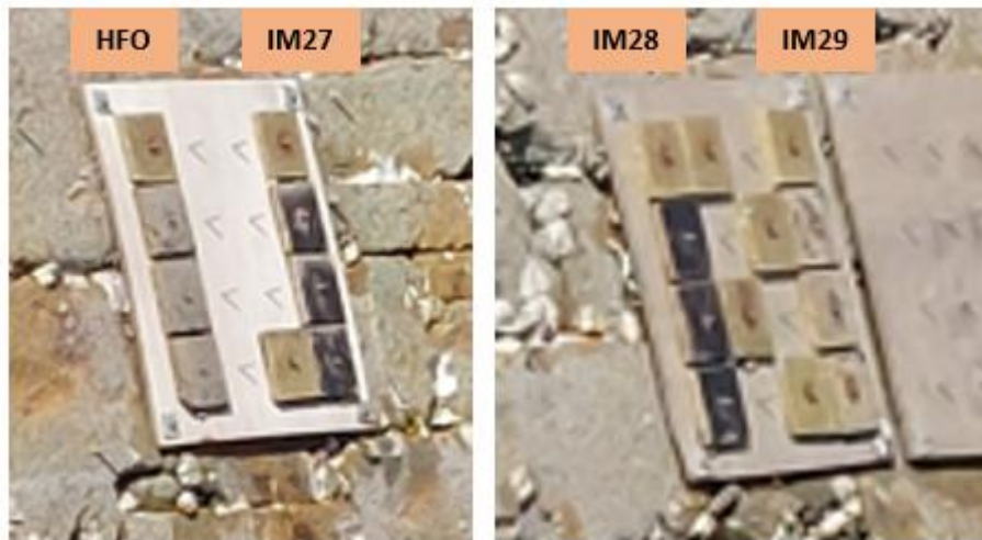
Figure 55 Pictures of the wooden frames installed on the South face of the quay, after 11 months of exposure
