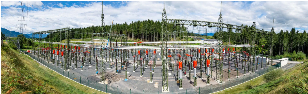
Figure 11. The Westtirol Substation in Haiming (Tyrol, Austria) (Source: APG)
