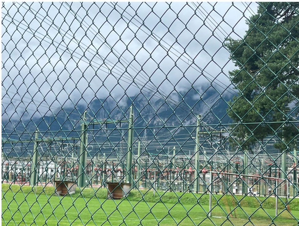
Figure 9. The electrical substation of APG in Haiming
