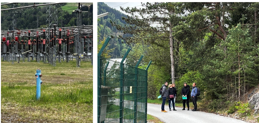
Figure 16. Water pumps in case of a fire(left) and snapshot from our visit to the Electrical substation (right)
