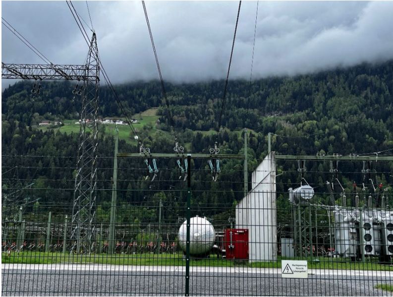
Figure 14. The electrical substation and the proximity to the forest
