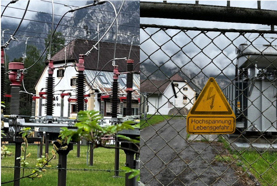
Figure 19. The TIWAG Substation
