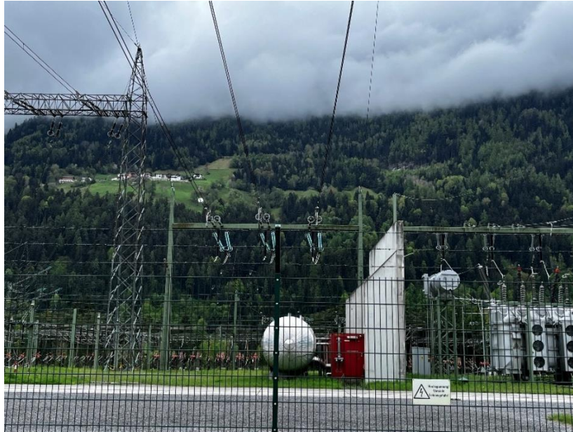
Figure 4. The electrical substation in Haiming.
